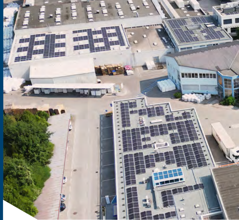
Photovoltaic systems at the Kremsmünster site
