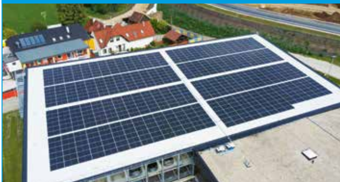
Photovoltaic equipment on roof of Greiner Campus car park in Kremsmünster
